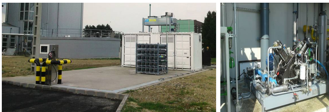
FIGURE 12: PHOTO IMPRESSION OF SMALL SCALE UPGRADING PLANT INCLUDING COMPRESSION TO 220 BAR, STORAGE AND DISPENSER.
